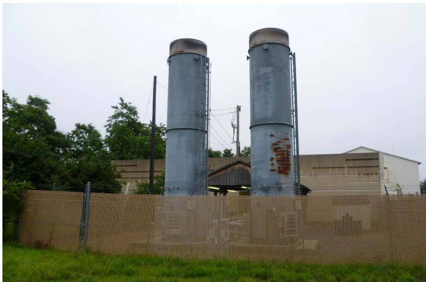
Figure A2. Large methane flares adjacent to the municipal landfill.
